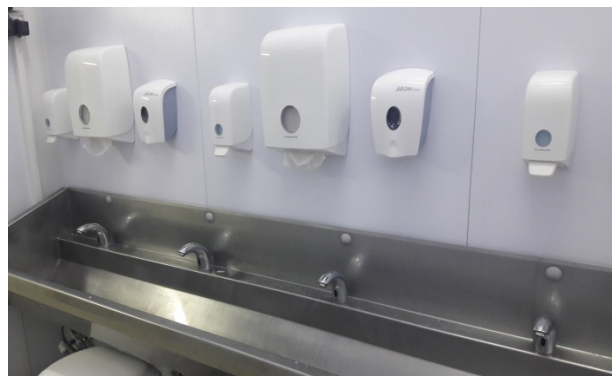
Figure 1. Contactless equipment for hand washing in final snails meat processing facilities
