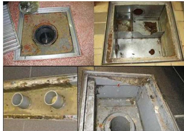
Figure 4. Poor drainage component design – metal to metal contact, gaps, sharp corners, non-drainable areas
